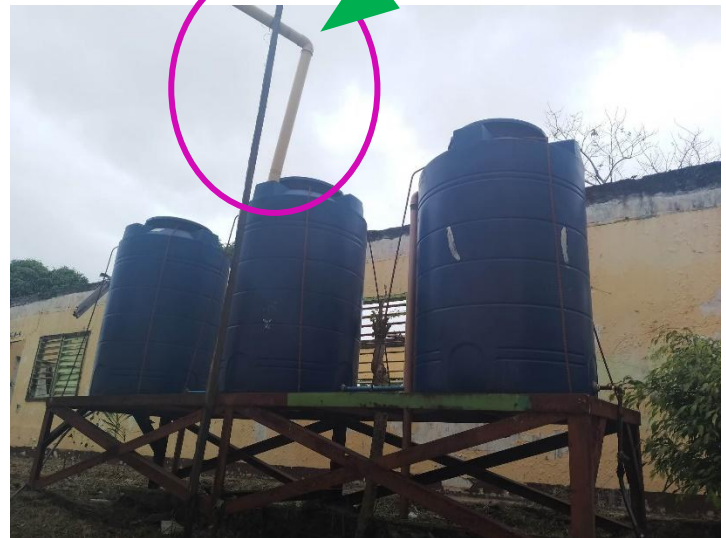
Water pipe from the Rain Catchers installed in the classroom roofs.
